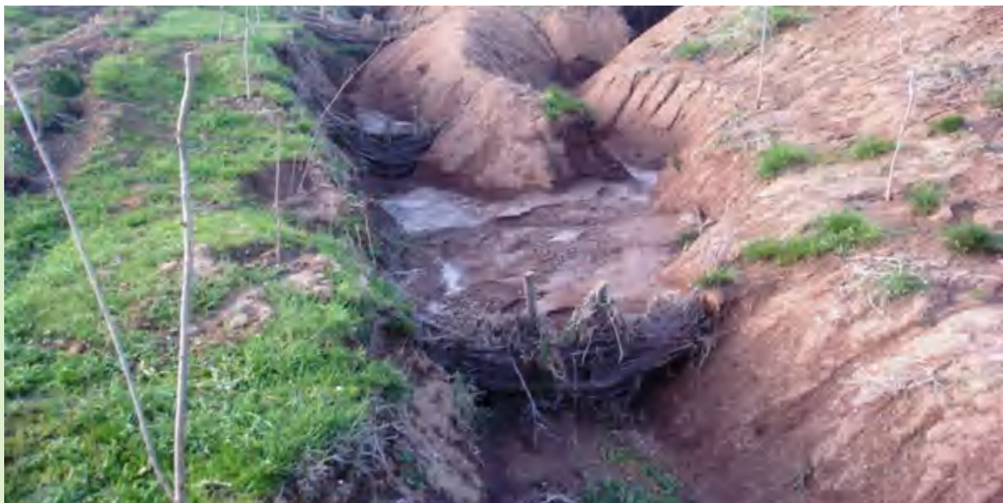
River erosion. ©Risha Solutions
