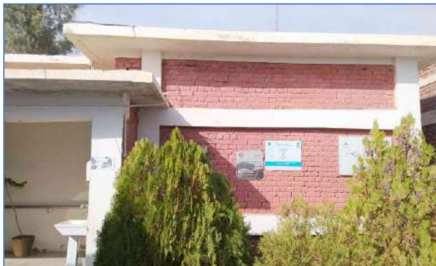
Plate 116: A view of after retrofitting of BHU at Killi Muhammad Khail, Panjpai, District Quetta.
