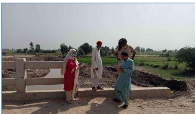
Plate 81: A view of consultation meeting with the sub-project contractor (HRC) regarding rehabilitation of old Deg Nullah at Bhudo Shahrif, District Shiekhupura.
