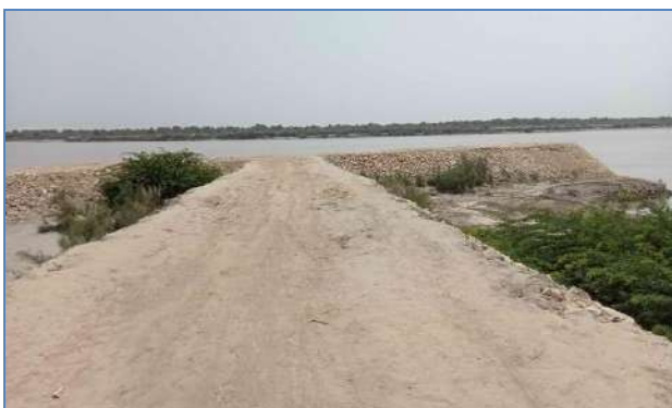
Plate 89: A view of re-constructed & recoument of damaged T-Head Spur at Agani Akil village, District Larkana.
