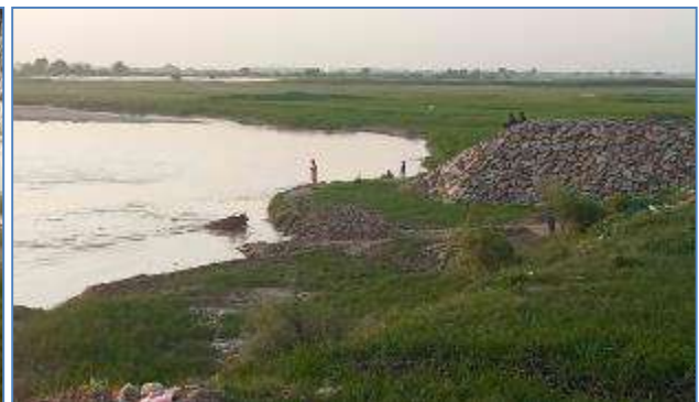
Plate 76: A view of constructed flood protection bund for protecting village Shahpur Chanjora, District Narowal.
