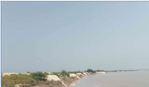
Plate 87: A view of constructed Stone Studs at Agani Akil village, District Larkana.
