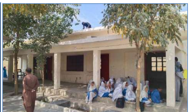
Plate 114: A view of after retrofitting school of Govt. Girls Middle School, Killi M Rehim, Kuchlak and Distirict Quetta.
