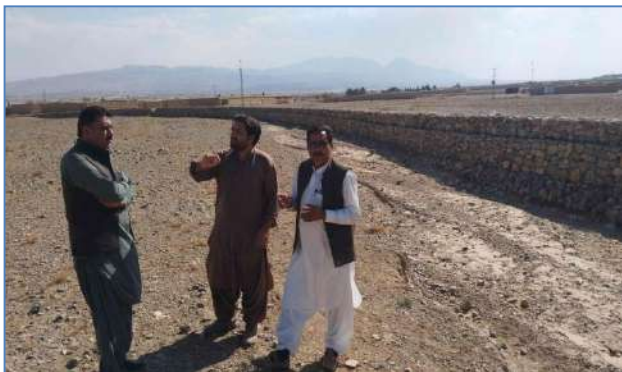
Plate 103: A view of Flood Protection Structure at Killi Regi Nasiran, Baleli and District Quetta.
