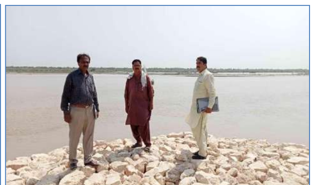
Plate 90: Site visit along with officials of Sindh irrigation department and view of constructed Mole Spurs at Agani Akil village, District Larkana.
