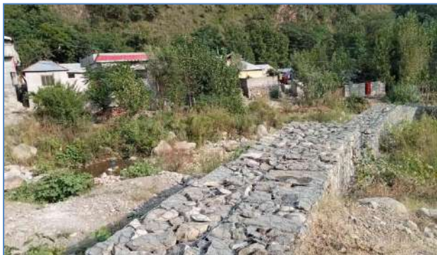
Plate 63: A view of constructed gabion protection wall at Bagh City, Nullah Mal, District Bagh.
