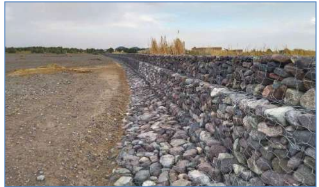
Plate 124: A view of after flood protection wall at Killi Azat Khan Nalap, District Chaghi.
