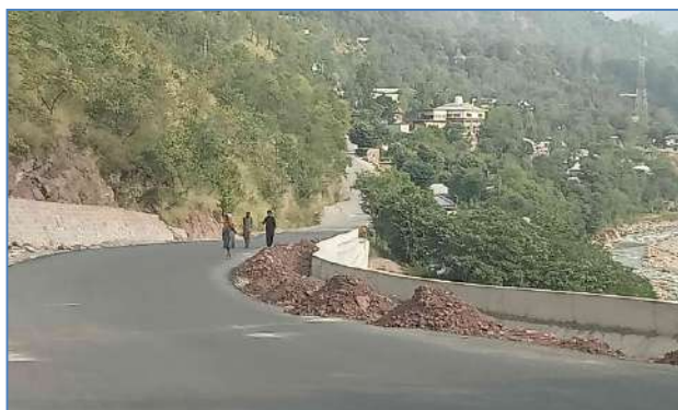
Plate 59: A view of constructed landslides protection wall at Arja, Teh Harighal, District Bagh.
