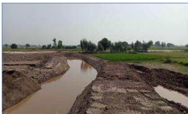
Plate 77: A view of rehabilitation of old Deg Nullah at Bhudo Shahrif, District Shiekhpura.
