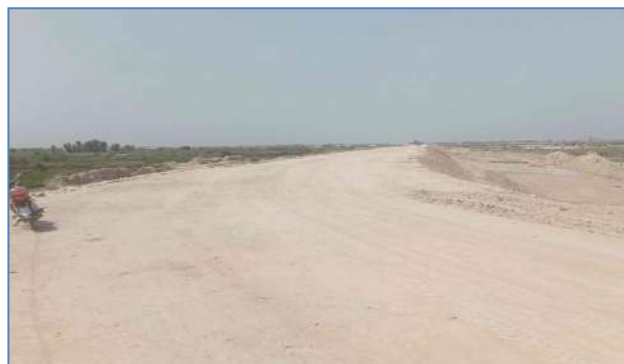
Plate 93: A view of re-constructed stone apron, stone pitching and earth work at Goth Shar Muhammad Bakarani, District Larkana.
