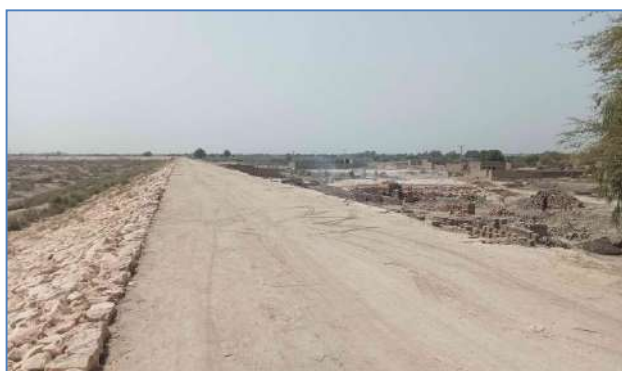
Plate 95: A view of re-constructed stone apron, stone pitching and earth work at Goth Shar Muhammad Bakarani, District Larkana.
