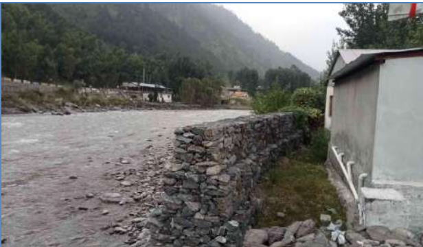
Plate 33: A view of Protection Wall at Hassa Pull, village Garlat, District Mansehra
