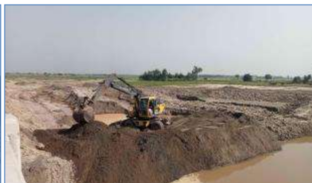
Plate 82: A view of rehabilitation work carried out of old Deg Nullah at Bhudo Shahrif, District Shiekhupura.
