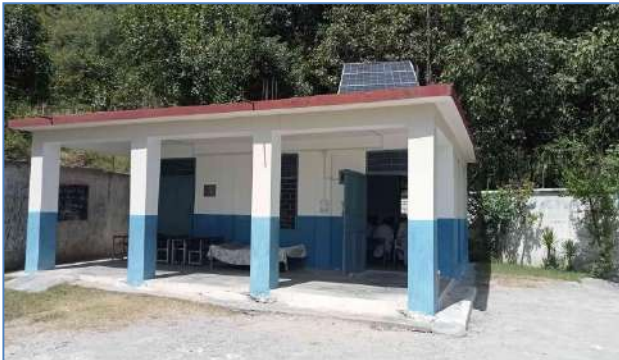
Plate 39: A view of after retrofitting school of GPS at Chita Batta, Bhogrmong and District Mansehra.
