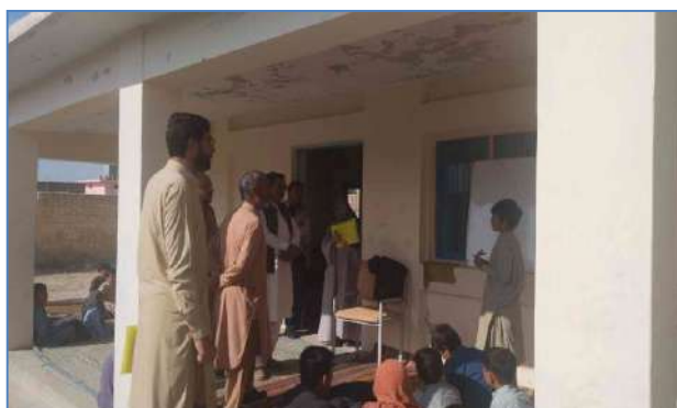
Plate 108: A view of after retrofitting School of Govt. Boys Primary School at Killi Kateer, Kuchlak and District Quetta.
