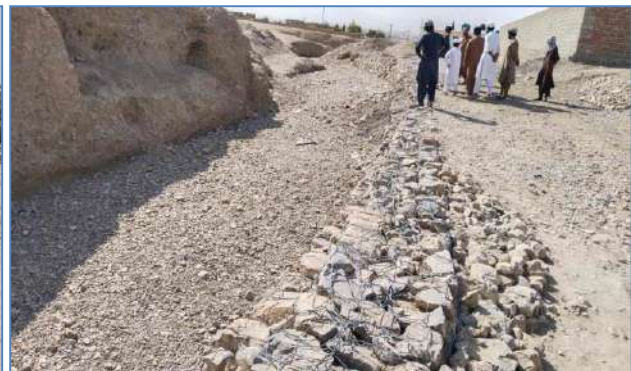
Plate 112: A view of after constructed flood protection structure at Killi Ragha Kakar Town, District Quetta
