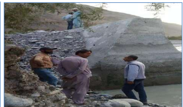
Plate 24: A view of flood protection wall at Gircha valley 1 and 2, District Hunza.
