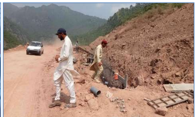
Plate 66: A view of landslides protection wall is in progress at at Azad pattan, District Pouch.
