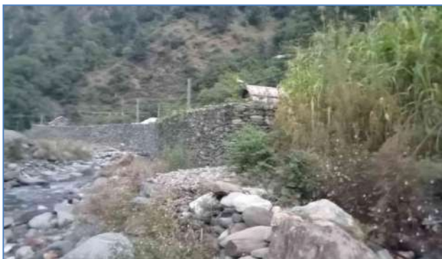
Plate 57: A view of constructed gabion protection wall at Leswa Bypass, Bhandi Ashkot, Teh Athmuqam, District Neelam.
