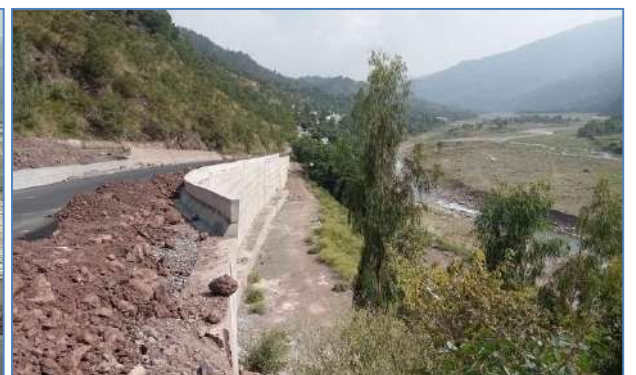
Plate 60: A view of constructed landslides protection wall at Arja, Teh Harighal, District Bagh.
