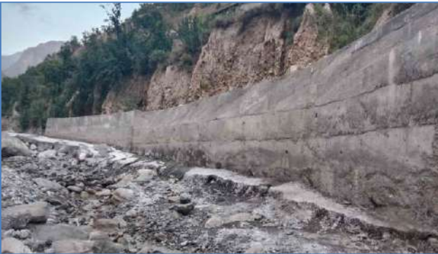
Plate 45: A view of constructed Protection Wall at Bokhtoli, Garam Chashma Valley, District Lower Chitral.
