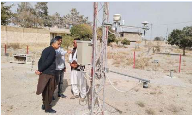
Plate 111: A view of installed early warning system at Pakistan Metrological Department Quetta.
