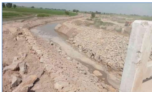
Plate 83: A view of rehabilitation of old Deg Nullah at Bhudo Shahrif, District Shiekhupura.
