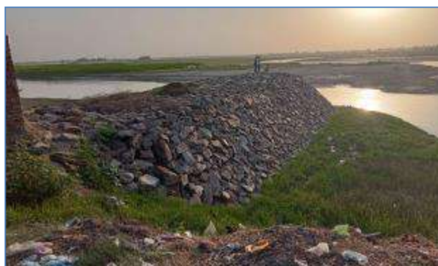
Plate 71: A view of constructed flood protection bund at Hajipur Gujran, District Narowal.
