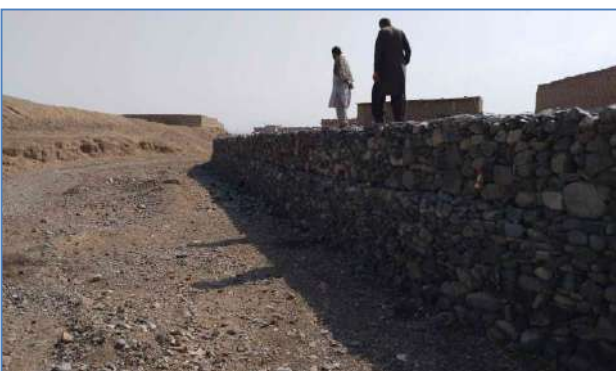
Plate 125: A view of after flood protection structures at Faisal Colony, Tehsil Dalbandin and District Chaghi.
